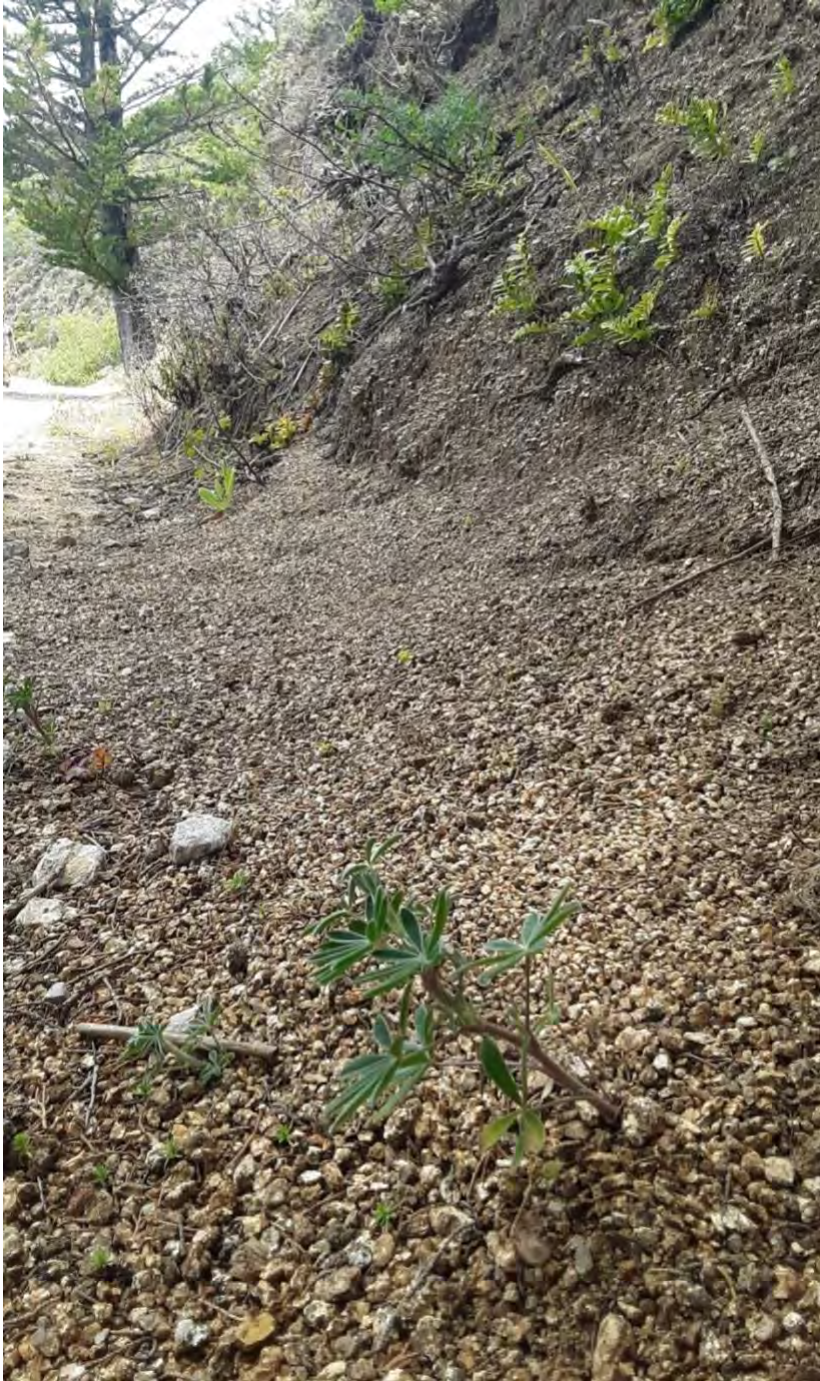
Figure 3: A new lupine sprout, potential host plant for the endangered mission blue butterfly, growing in the sloughing decomposed granite along the roadway, material that will be used to fill rills, ruts and gullies in the roadway.
