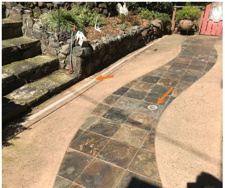
PHOTO 4: Trench drain and patio drains at front entry patio
